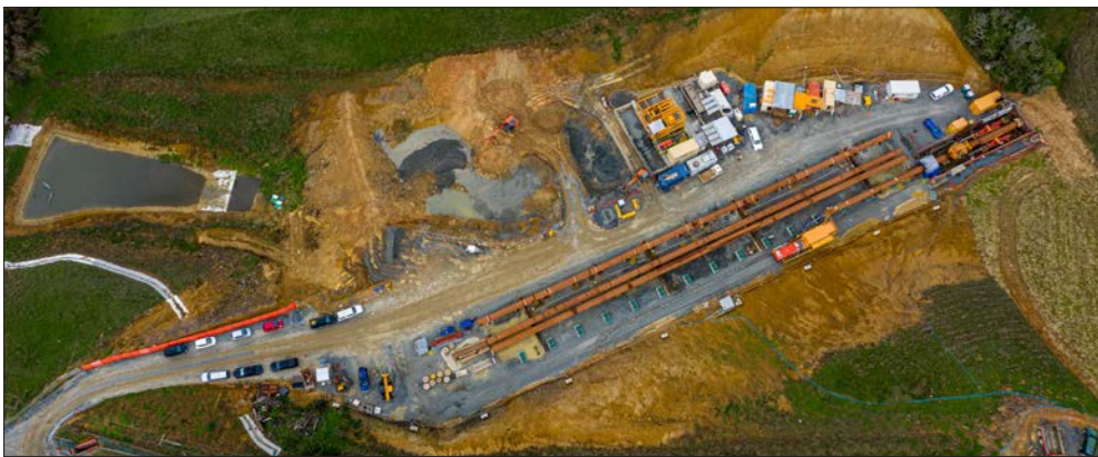
Above and opposite: McConnell Dowell set a new World Record on Watercare's Snells Algies Ocean Outfall project in New Zealand for Herrenknecht's Direct Pipe technology with a drive of 2.021km.
